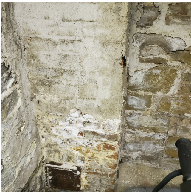
Interior Stone Foundations with Efflorescence
