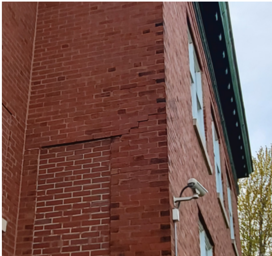
Cracks above In-filled Windows Due to Lintel Corrosion
