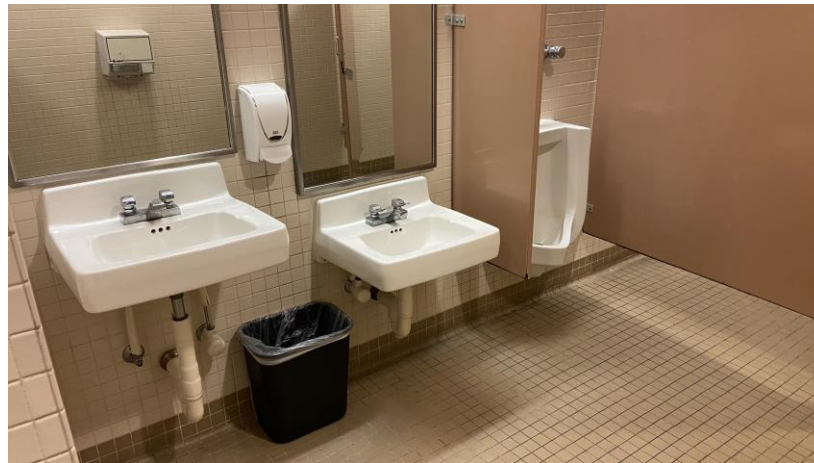
Fig. 23 - public restrooms with older fixtures and spring-actuated faucets.
