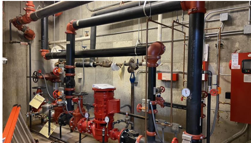
Fig. 24 - incoming fire protection service, fire pump, backpressure prevention device, and pump controller.
