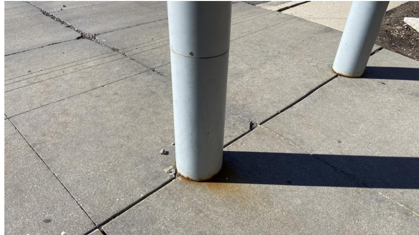
Fig. 2- Corroded light bollard bases.
