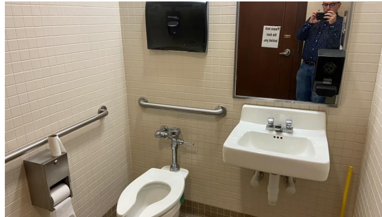
Fig. 7- Inadequate side transfer space and rear grab bar length.
