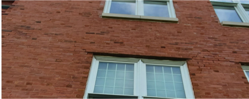
Cracks above Windows Due to Lintel Corrosion
