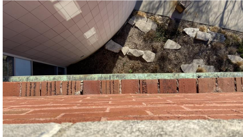
Fig. 11 - mortar loss as viewed from Carnegie portion roof
