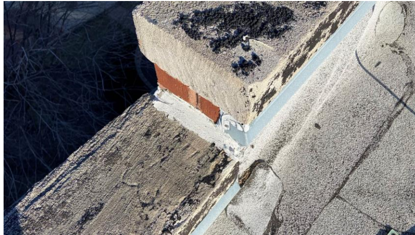
Fig. 14 - stone cap degradation and black residue observed in several locations.
