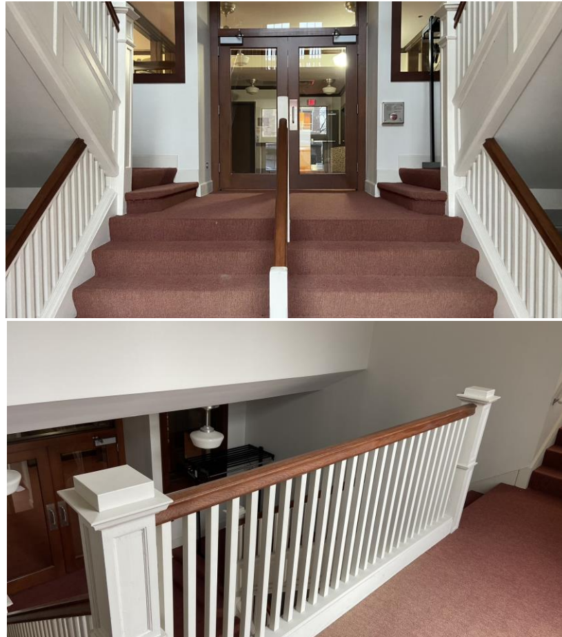
Fig. 9 & 10 - non-compliant handrails and guardrails at original portion of building.
