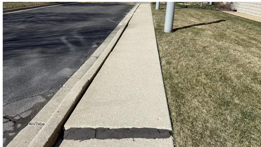
Fig. 3- Damaged/cracked sidewalk areas.
