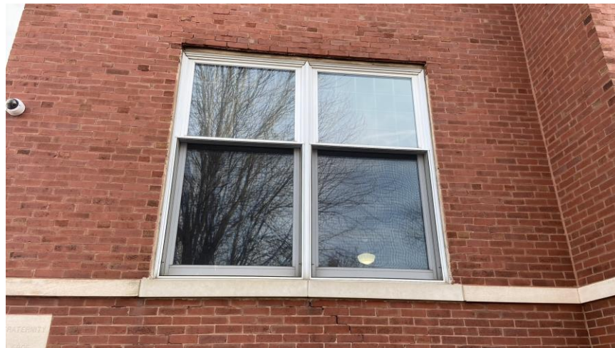
Fig. 5- Example of masonry damage and lintel corrosion above window in Carnegie portion of building.
