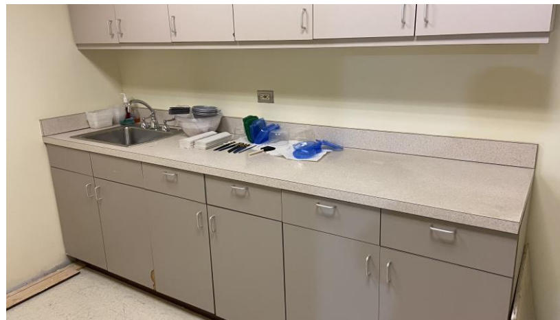
Fig. 8 - Lack of knee space at staff and public area sinks.
