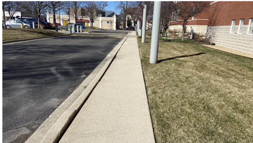
Fig. 1- Sidewalks separated from curb, resulting in large gap and level change at curb.
